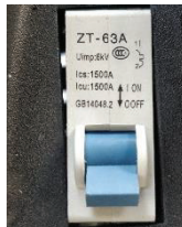
2. MCB is turned OFF
